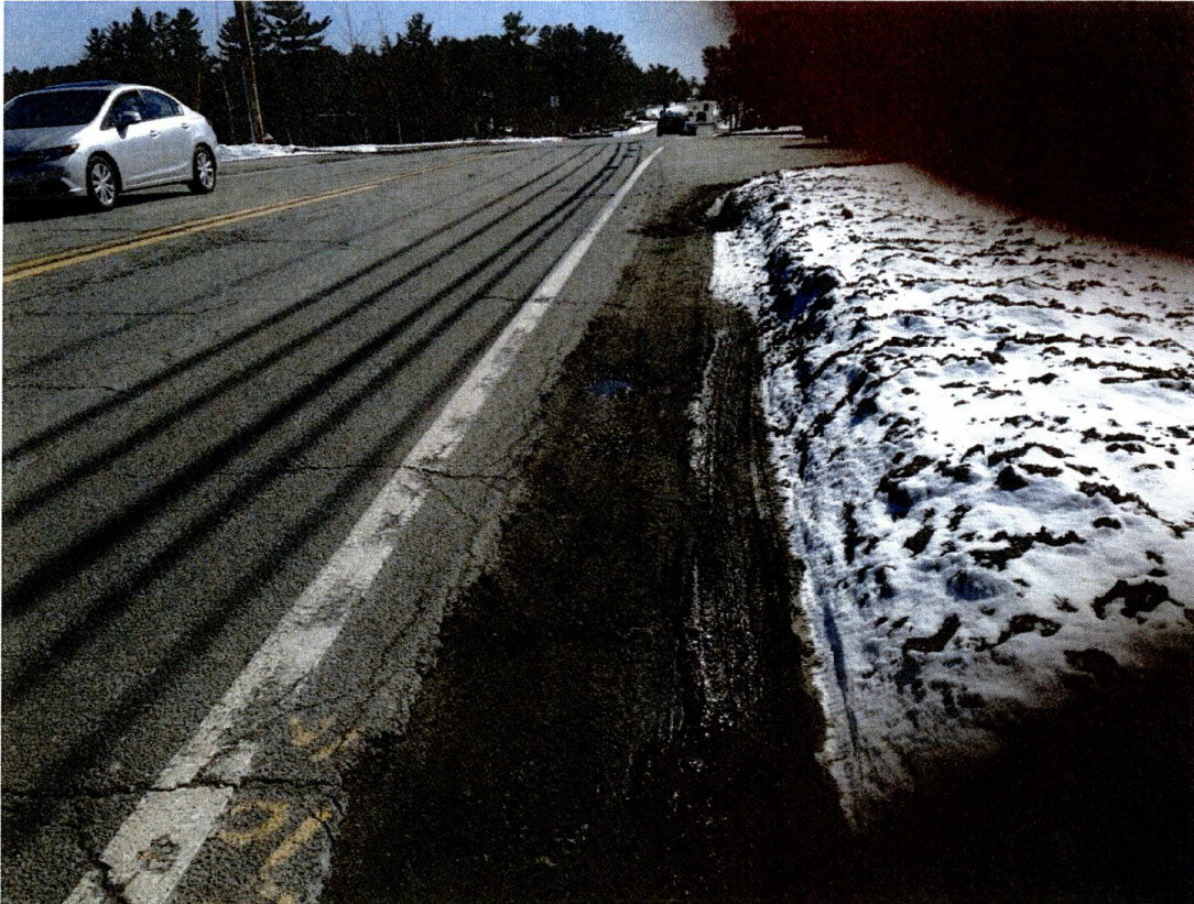
Photo 2 – Southbound Shoulder Damage
